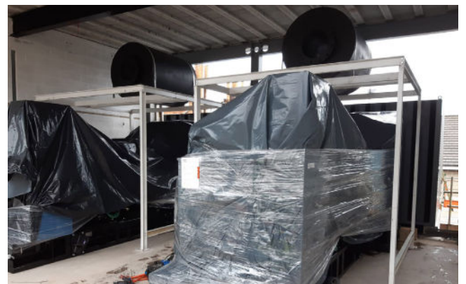
The proposed generating sets were carefully selected by the WB Power estimating team, following a detailed analysis of the Hospitals requirements. WB Power were able to strike a careful balance of fuel efficiency, upfront costs and ongoing service requirements.
