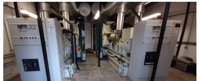
As part of the installation, the incumbent plant room had all its equipment removed and some remedial civil works were then completed prior to the new installation commencing.
